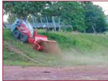
Bozena in operation
