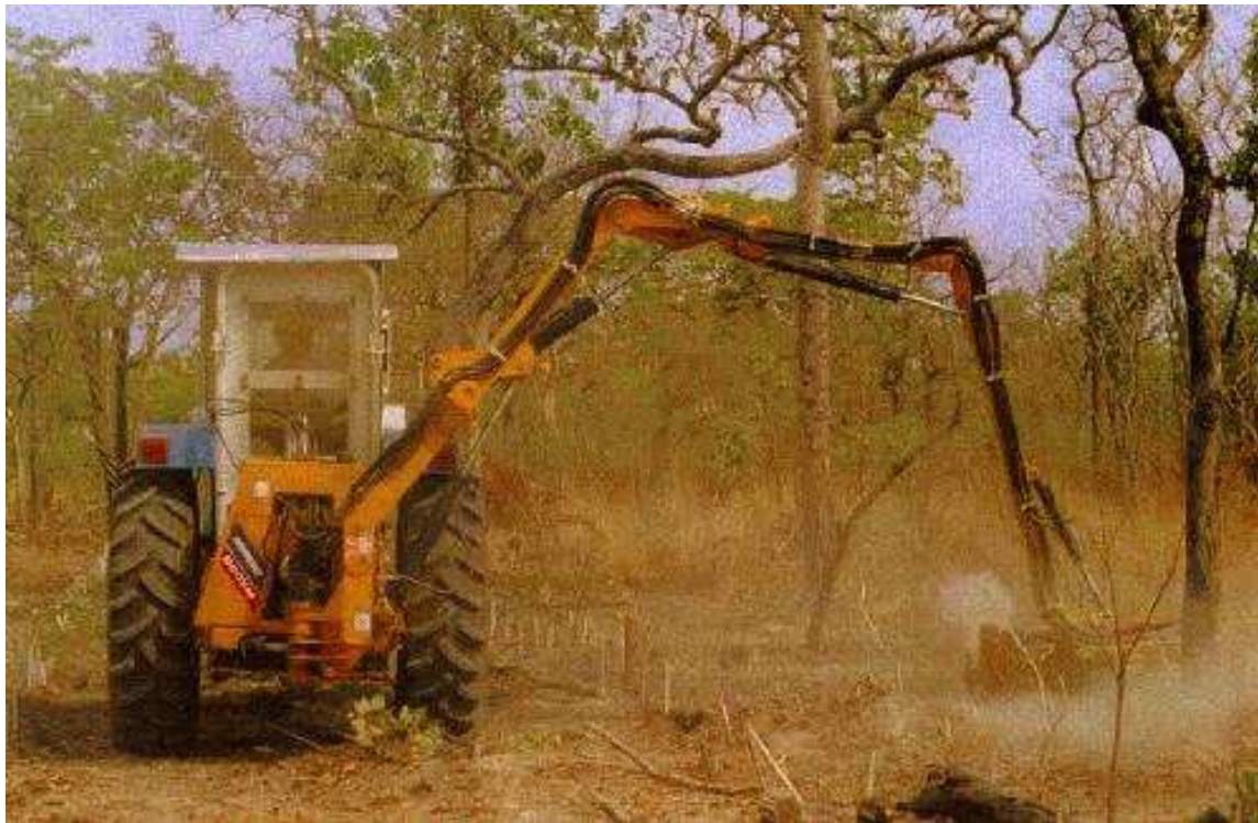
Figure 2.3: Vegetation clearance using a flail on a long boom on an armoured tractor. Note: tractor and cab are heavily armoured on right-hand side only. From CD-ROM catalogue of demining equipment [M + 99].
